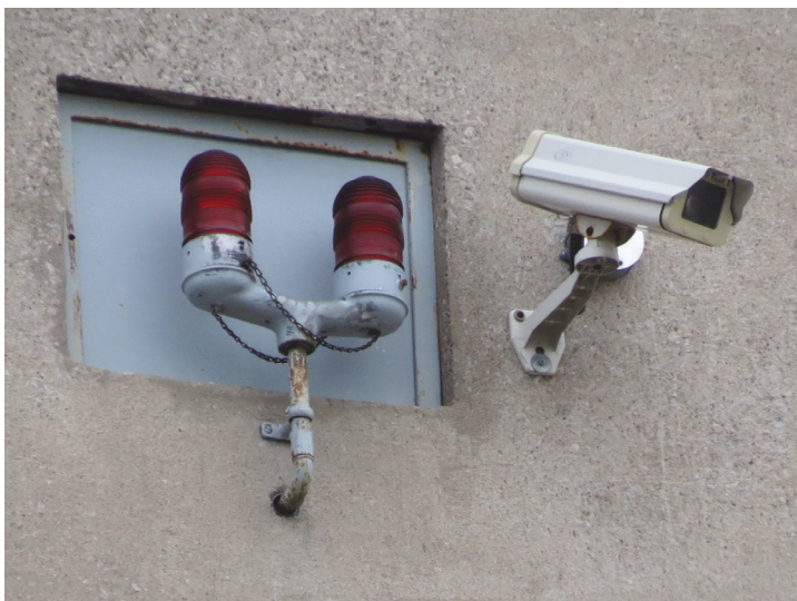
Fig. 17 A photograph of the aircraft warning lights and security camera as mounted on the side of the York University Stack
